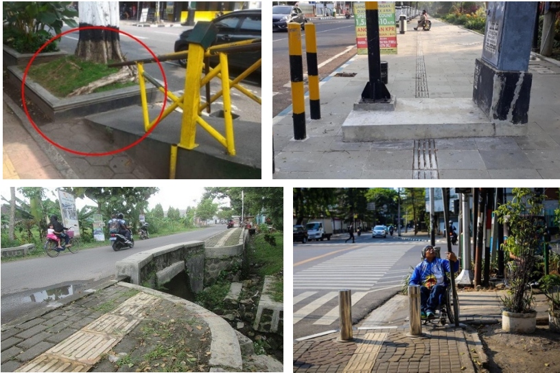
Figure 1. Four examples of sidewalks design in Indonesia cities which barely accommodate the need of the disabled, i.e., a steep ramp with blocking end, discontinued guiding blocks and narrow space for those with wheelchairs
